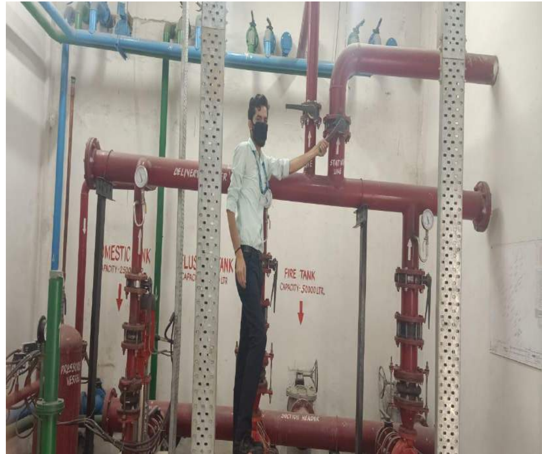
Date – 24-04-2020 , Place- Fire pump panel, GNIDA Station, Greater Noida
